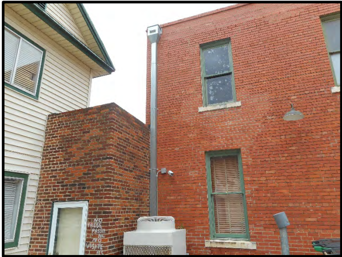
Rainwater gutter at 204 S. Oakes St. (to connect to new rainwater building)
