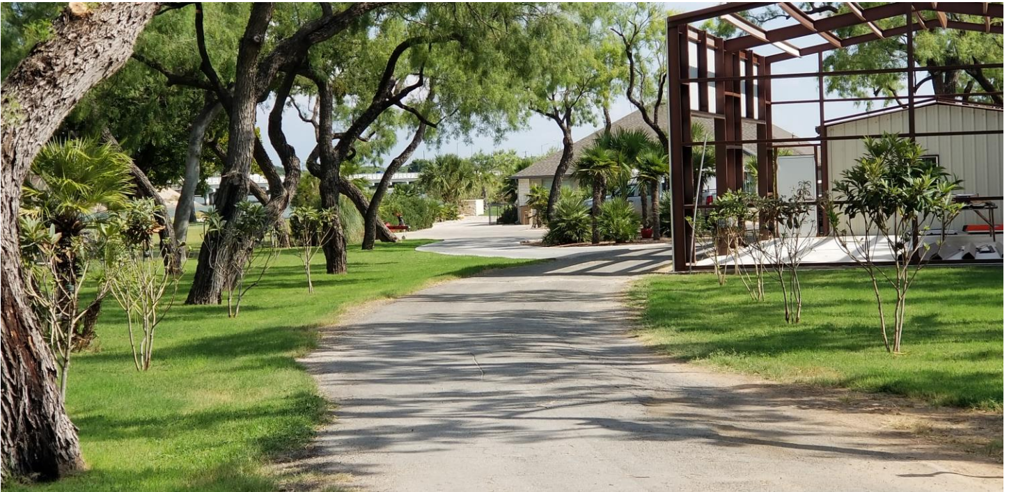
Close up of the relationship of the new garage to the house and the existing garage.
