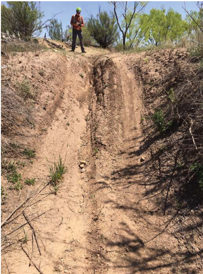
Eroded approach into channel in motorcycle trail area
