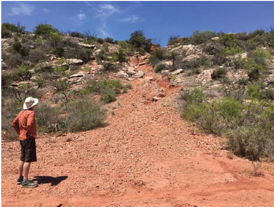
Alluvial deposit from eroded crawler trails in “The Bowl”
