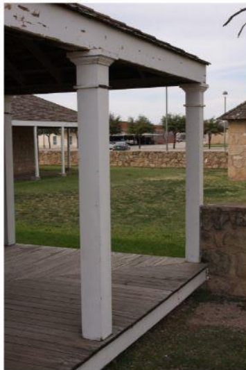
PAINT COLORS WILL MATCH EXISTING COLORS AND PAINT LOCATIONS. ROOF OVERHANGS ARE BEING EXTENDED TO MATCH HISTORIC PHOTOGRAPHS AND HELP TO PROTECT THE WOOD COLUMNS
