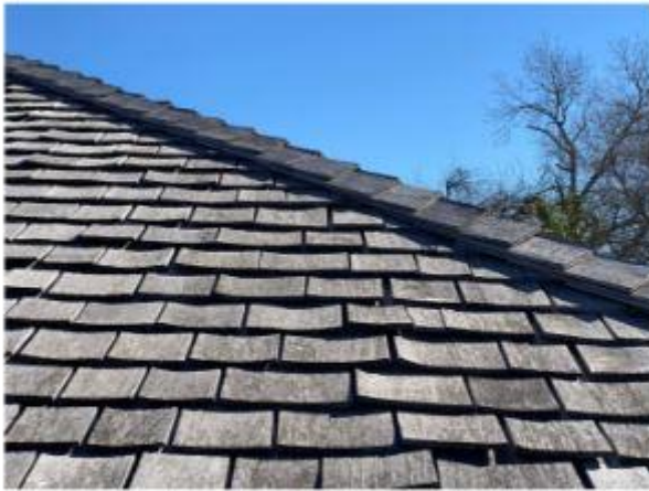
WEATHERED WOOD SHINGLE ROOF
