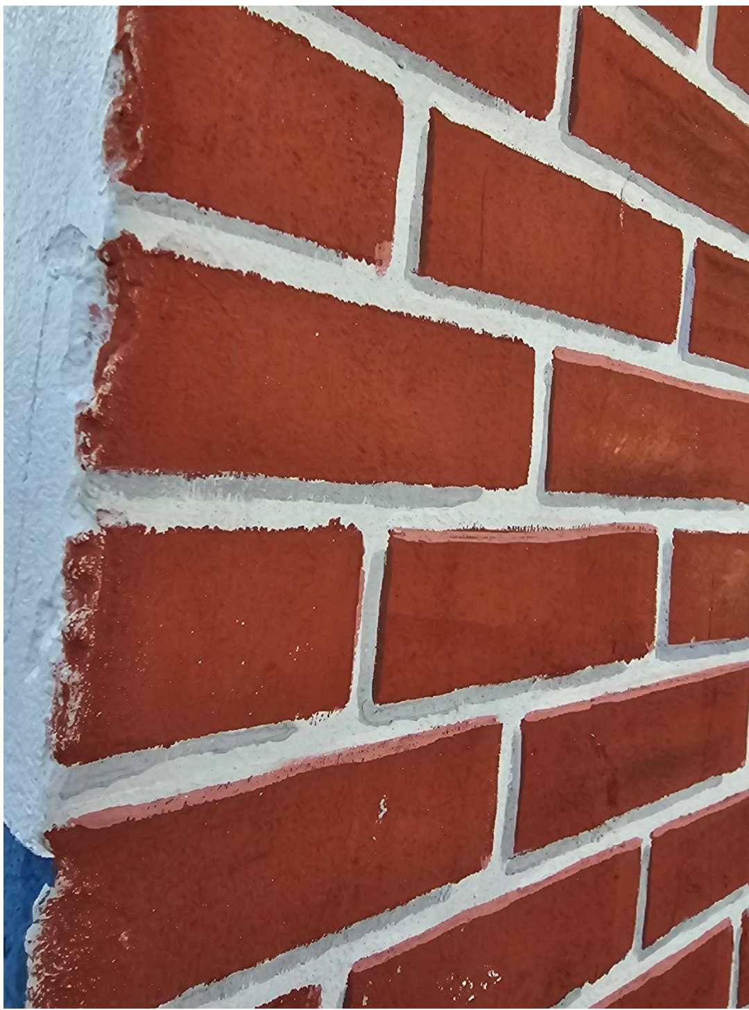
The stucco wall that covers the existing bricks that are to be cleaned and restored.
