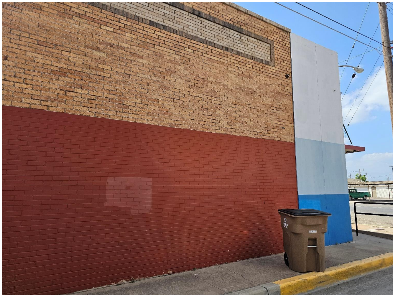
Showing the painted brick that we hope can be restored and the site to the right that shows where the art will be painted (on the white area).
